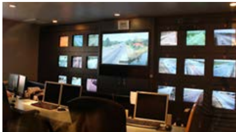
Figure 3-9: Traffic Management Center in Boise, ID (Source: Noblis 2012)
